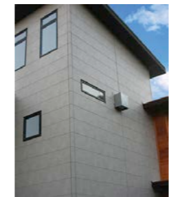
A Nichiha style panel system will be used with a strong horizontal proportion on the sides and back of the building to give the home a long low look.
